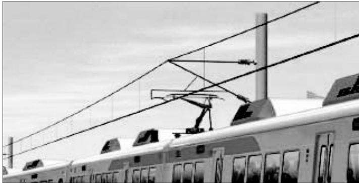
Figure 14 - Overhead Traction Supply System
